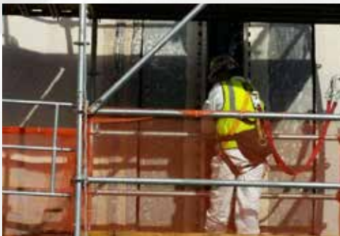
Installation of duct flanges and tee beams for scrubber rebuild during a smelter shutdown 🔄
